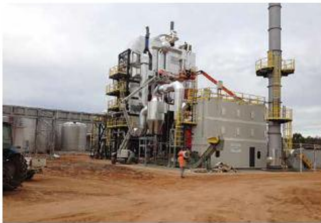
The Australian Tartaric Products Biomass Power Plant's boiler at 80 per cent completion.
