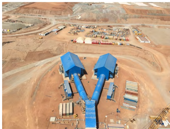
Shaft 2 Mine Air Heater Houses commissioned October 2019, to support up to 200km's of underground tunnels (1.3km's below the surface)
