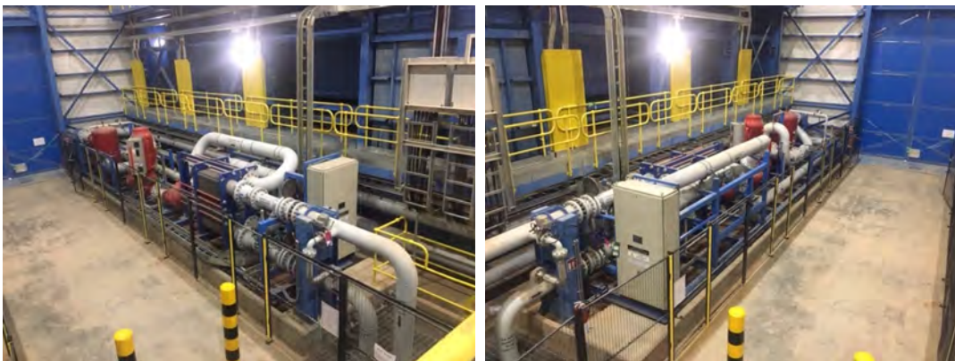
Heat transfer stations inside shaft 2 heater house
