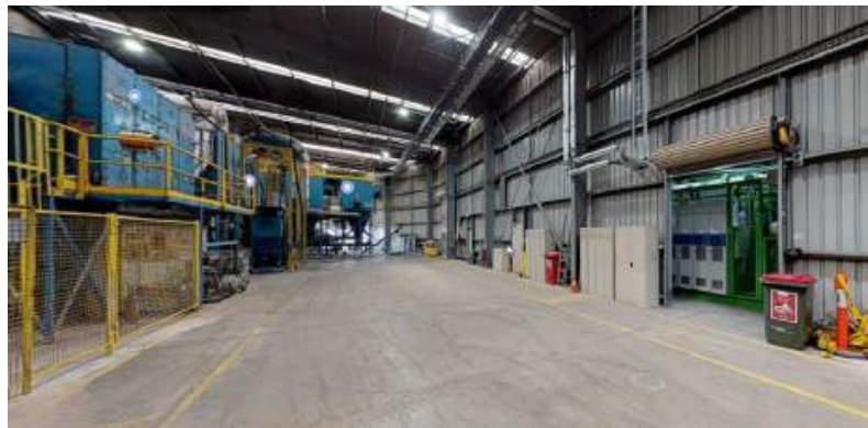
gTET ORC Generator in position at Veolia. Insulated hot water pipes can be seen from the EGHX to ORC.
