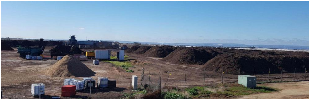
Jeffries site, prior to the pyrolysis and power station installation, showing the biomass fuel storage.
