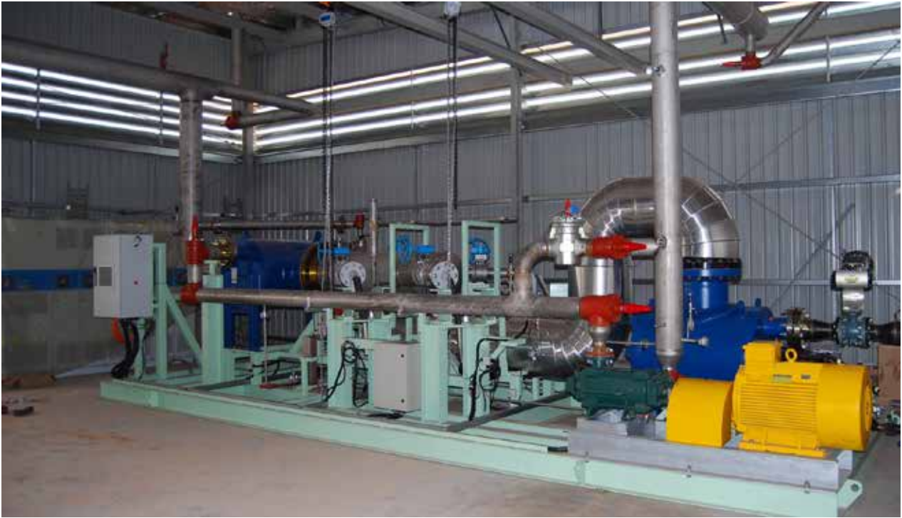
gTET's 600kWe ORC generator comprising 4 high speed turbo-alternators and integrated turbine drive and grid inverter (far ground)
